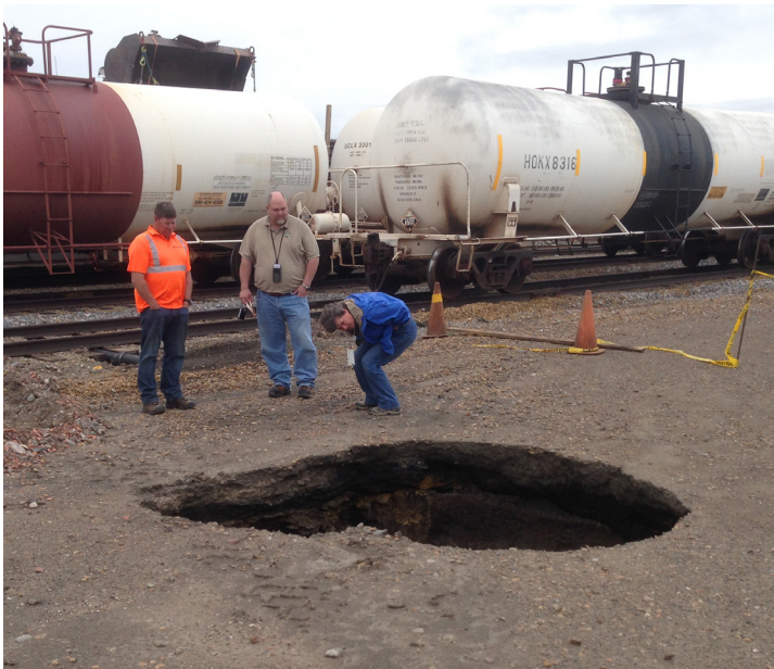
Sinkhole southeast of Dickinson
